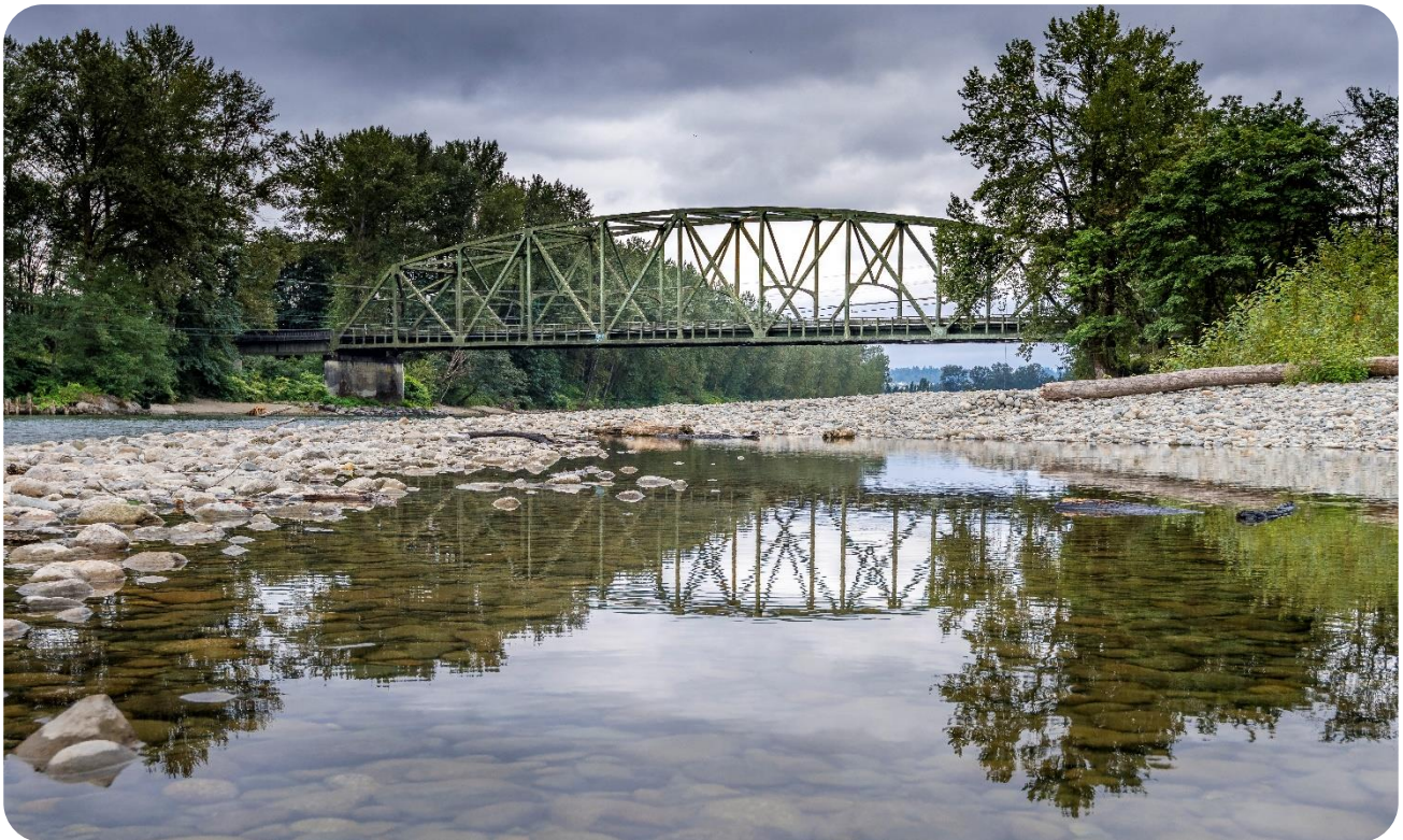
Skykomish River Bridge Source: Provided by the City of Monroe, Credit to Dan Evans
