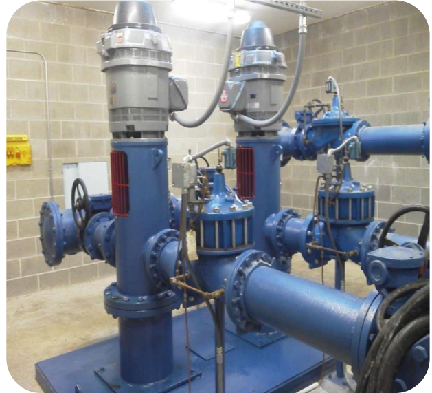
Tester pipes Source: City of Monroe
